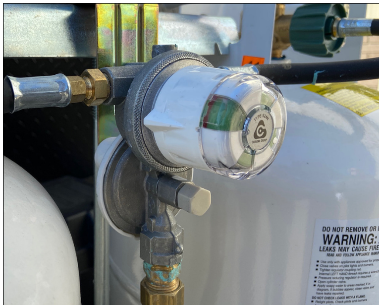
FIGURE 16-5: A pressure regulator and crossover valve on a typical dual tank system.
