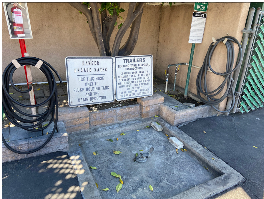
FIGURE 15-7: A public wastewater dumpsite.
