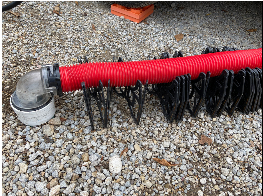
FIGURE 15-5: A “slinky” hose properly connected to a campsite sewer.
