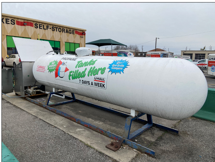
FIGURE 16-7: When you're hunting for a propane fill-up, look for a big horizontal tank shaped like a giant Tylenol capsule with some pump equipment at one end.
