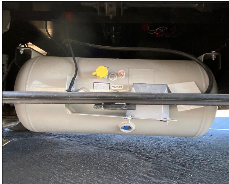
FIGURE 16-6: A permanently mounted ASME motorhome propane tank contains an inlet valve and a built-in mechanical float gauge.
