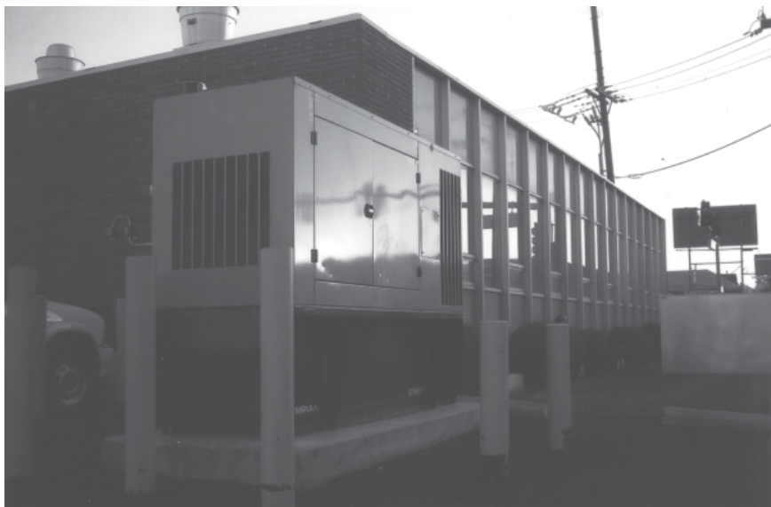
Figure 13-2. Emergency generator. ( Photo by Robert Reid, 2004. )
