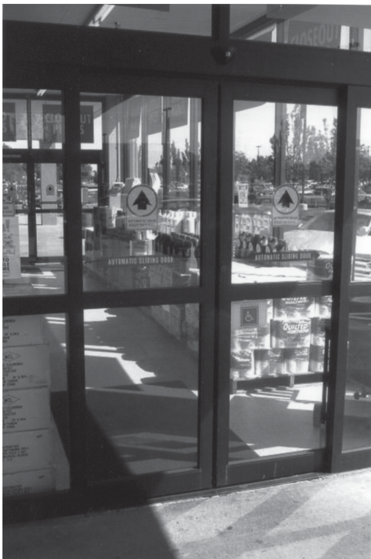
Figure 5-5. Sliding glass door. (Photo by Robert Reid, 2004)
