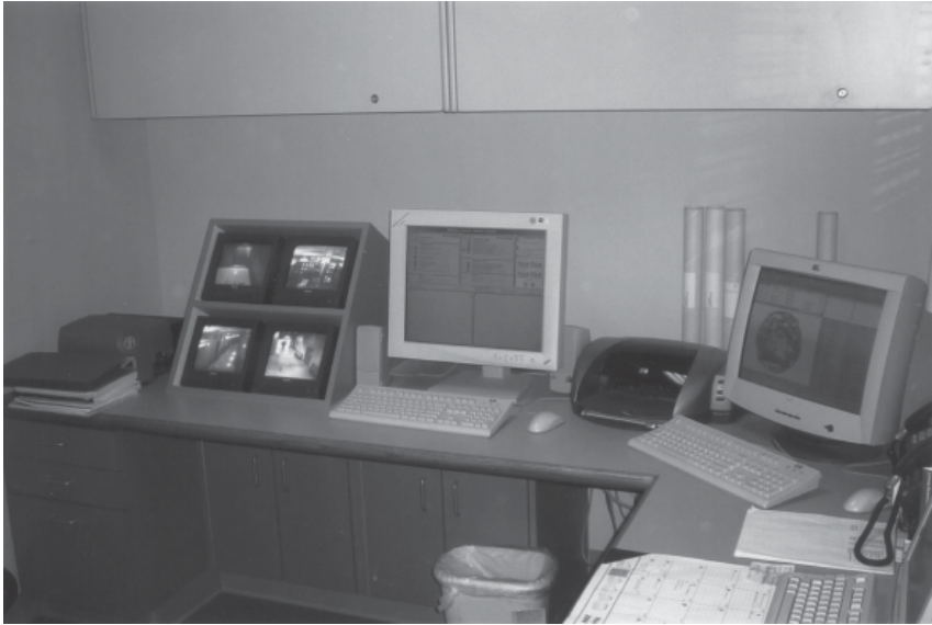
Figure 9-3. Control room station. (Photo by Robert Reid, 2004)
