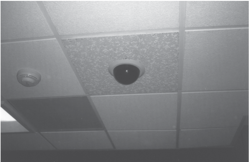
Figure 11-1. Indoor dome camera. (Photo by Robert Reid, 2004).
