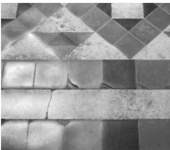
Figure 5.29 Damage forming a trip hazard in floor tiles at the entrance to a church.
