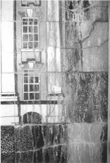
Figure 5.16 Severe surface pollution.
