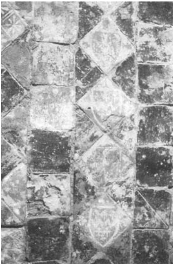
Figure 5.8 Lime encrustations on medieval tiles.
