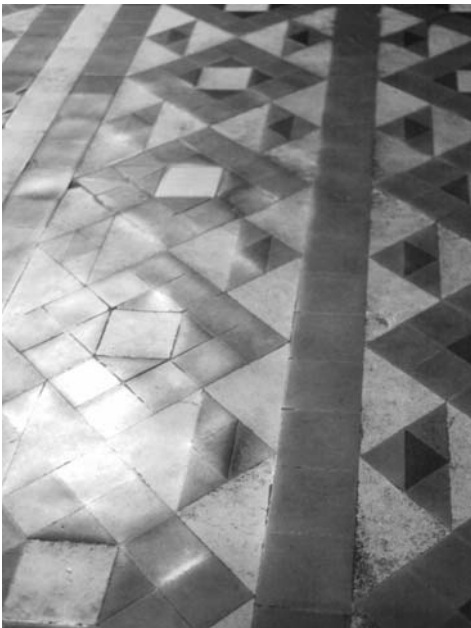
Figure 5.4 Typical damage caused by tread.
