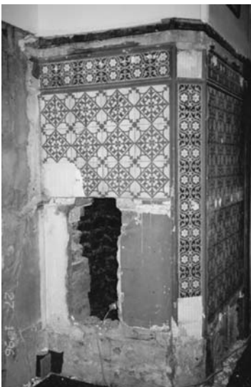
Figure 7.13 Damage to scheme caused by the letting in of heating ducts to walls.
