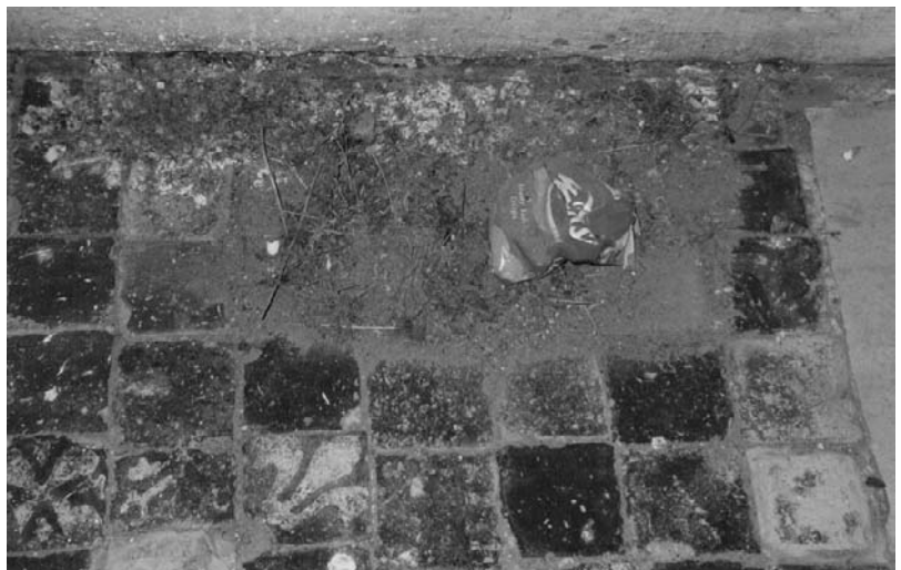
Figure 5.7 Debris on medieval tiles underneath a nest site.
