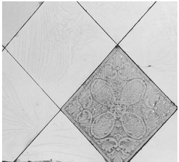
Figure 5.5 Typical crazing on old glazed tiles.
