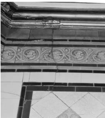
Figure 5.6 Fracturing caused by building load.
