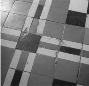
Figure 5.21 Spalled edges of tiles due to tensile pressure.
