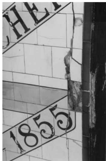
Figure 5.25 Compressive tension and shifting causing fracturing and misalignment.
