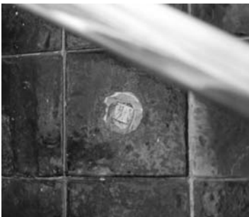
Figure 5.32 Steel fixings left in glazed tiles.
