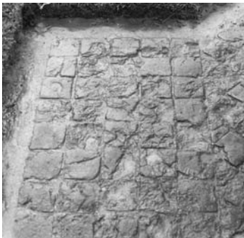
Figure 7.19 Frost damage on tiles, the result of many years' exposure.
