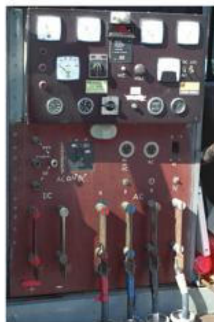
FIGURE 8.5 The output panel on a generator.
