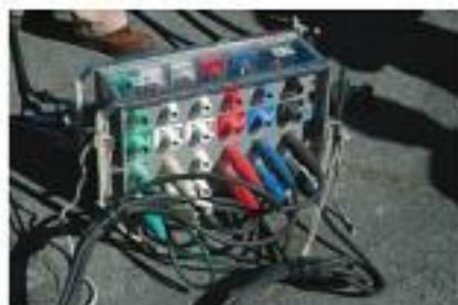
FIGURE 8.9 A connector box such as this makes the use of “threeefers” or “tees” unnecessary and thus simpler.
