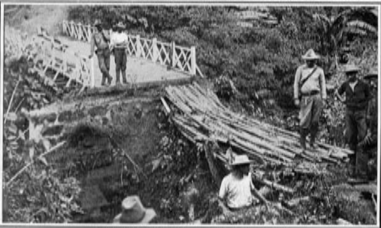
The Destroyed Bridge near Hail, which was blown up by Filipinos in Hailcoat THIS SHOWS THE EFFICIENCY AND RESOURCEFULNESS OF OUR ENGINEERS IN REPAIRING IT FOR SERVICE
