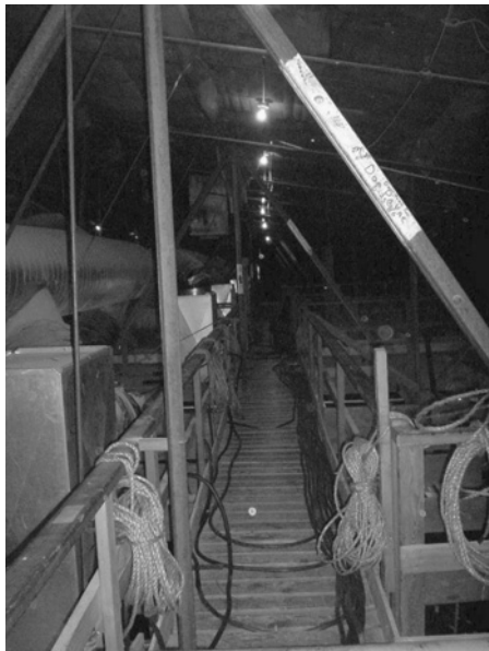
Figure 19.81 This is what the perms walk might look like when you are just starting the build day. By the time it is ready, it will probably be filled with a lot of electrical cables and other things. It gets very crowded up there. Be careful.
