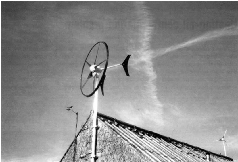
Figure 9.6 Swift rooftop wind energy system
