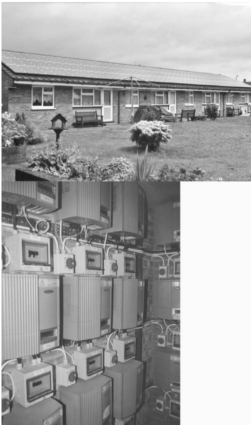
Figure 19.4 Prior's Croft PVs and inverters to convert DC power from the PVs to AC electricity
