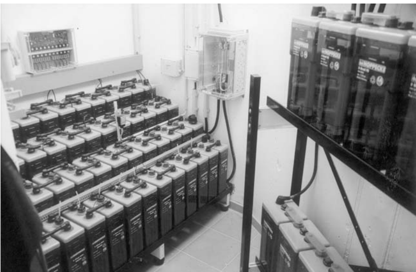
Figure 13.8 Banks of lead acid batteries in the Freiburg Solar House
